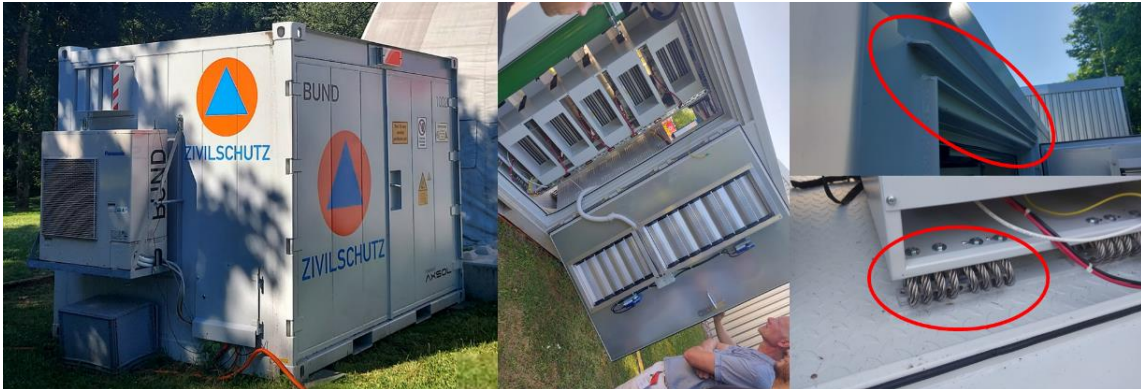
Figure 5: Features that stood out during the inspection included shock absorbers, drip edges, maintenance doors, and external components like air conditioning.
